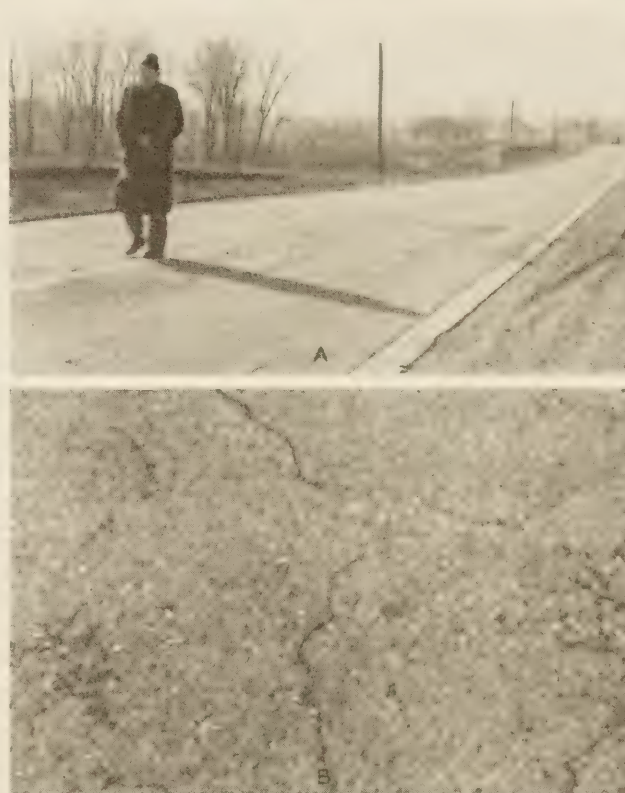
FIGURE 2.—A, GENERAL VIEW, AND B, SURFACE DETAIL OF A PAVEMENT THAT WAS RATED VERY POOR. NOTE THE SPALLING ALONG THE CRACKS AND THE RAVELED CONDITION OVER A LARGE PORTION OF THE PAVEMENT. SAMPLE S B WAS TAKEN AT THIS LOCATION. THE PATCHED SAMPLE HOLE CAN BE SEEN IN THE RIGHT CENTER OF THE UPPER PICTURE.
